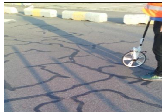
Figure 2 - Fatigue and low-temperature cracking
