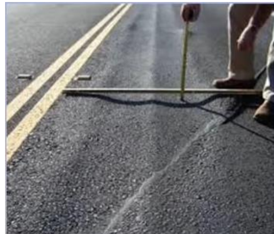
Figure 1 - Classical deformation (rutting)
