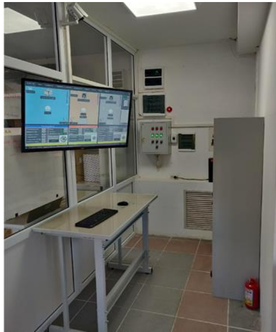
Figure 1. Control Room Configuration
