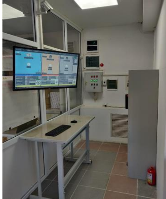
Figure 1. Control Room Configuration
